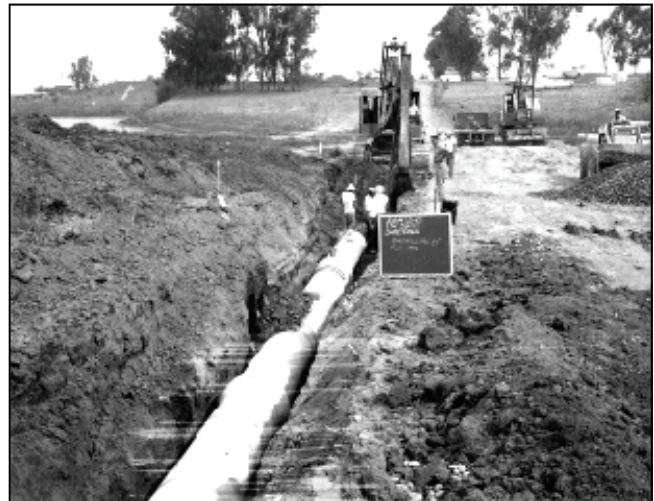
El Toro Water District employees laying water pipe at Moulton Parkway and Ridge Route in September, 1964.
