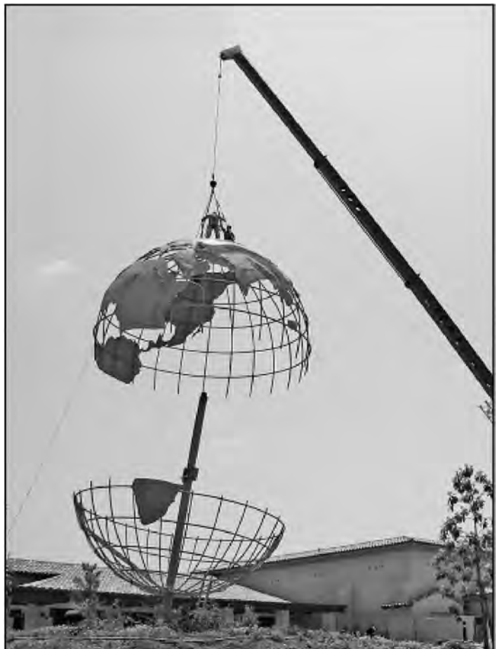
Picture 31 - Workman cut along the center of the Globe. Both halves, each weighing about one ton, were lifted to the parking lot. The next day the halves were cut up so that the steel could be recycled.
