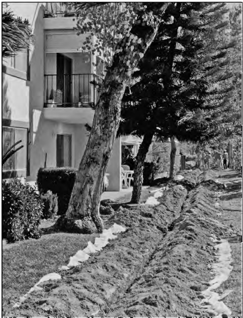
Picture 20 - In 1996, trenches were dug throughout the community so that fiber optic cable could be connected from the Head-End Building on Campo Verde to more than 2,550 buildings in Leisure World.
