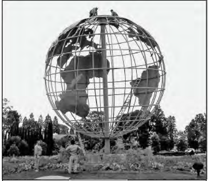
Picture 30 - In February 2002, workers prepared to move the Globe from Avenida de la Carlota to Moulton Parkway, next to Clubhouse VII.
