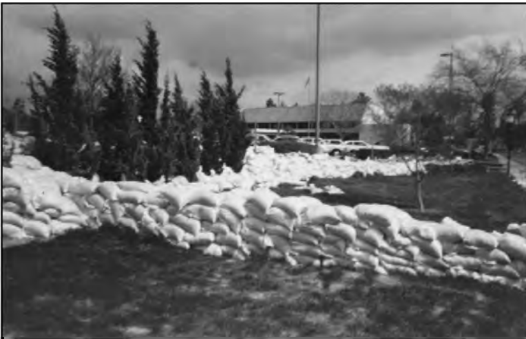
Picture 22 - Sandbags were used in an attempt to minimize water damage. Ultimately 24 inch high concrete block walls were installed to protect homes from future flood damage.
