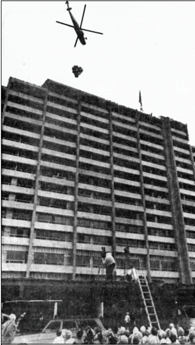
A 4,000-pound carob tree was lifted to the roof by helicopter April 20, 1974 at the "topping out" ceremony celebrating completion of the frame of twin 14-story condominiums at Rossmoor Leisure World in Laguna Hills. San Francisco Mayor Joseph Alioto spoke at the event, attended by some 3,000 people. The Rossmoor Towers flag was also hoisted to the top of the building and blue and white balloons and white doves were released at the end of the ceremony.
