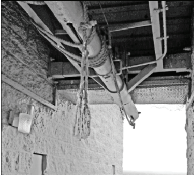
Remains of the rope crane used to hoist furniture into units until it was declared a safety hazard in the 1980s.
