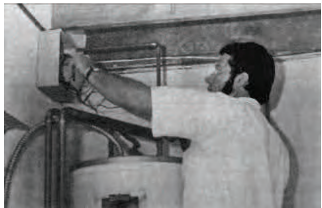
In October, Southern California Edison electricians began installing devices on community water heaters and air conditioners as part of experimental "automatic powershift" program. Through the electronic devices, the appliances will be shut off for short periods of time on days when energy demand is at its peak. Devices were to be installed in all manors by June 1978.
