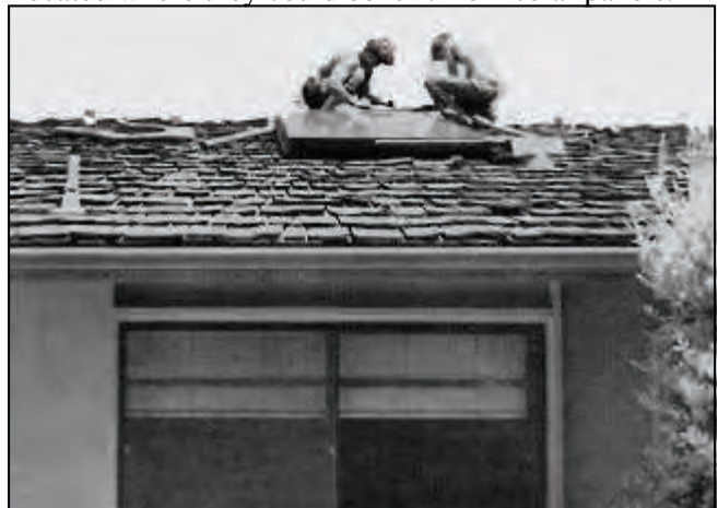
The first Leisure World manor went solar on August 25, 1979. One large smoky glass solar panel on the roof of Mr. and Mrs. Walter Bott's manor provided enough hot water for everyday chores. Mrs. Bott reported that the system provided water sufficiently hot for dishwasher and showering. “But wouldn't you know it,” she commented, “the first day I washed clothes, it was cloudy.”
