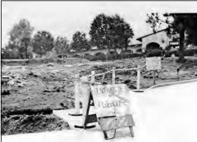
Early in 1978, GRF constructed the circular driveway that allows passengers and equipment to be dropped off at the entrance to Clubhouse II.
