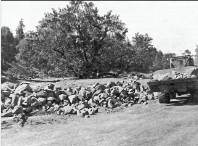
In danger of being surrounded by water if there was another onslaught of heavy winter rains, the decision was made to surround the 450-year-old sycamore in Aliso Creek with huge boulders. Leisure World News
