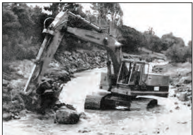
Backhoe fortifies the banks of Aliso Creek in February 1980, in an attempt to prevent further erosion.
